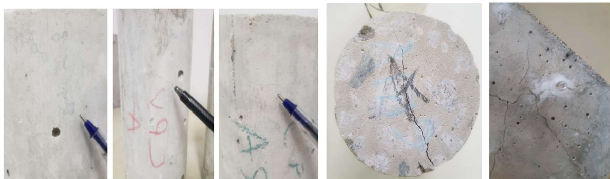
Figure 16 – Visual inspection – surface ASR effects on specimens
